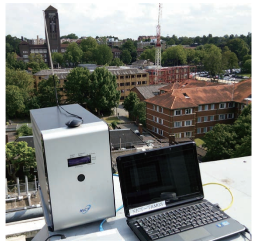
■ Figure 2: LTE base station installed on a roof in the university campus
