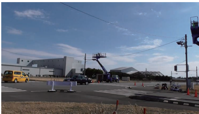
Figure 3: Measurement site with two roadside 79GHz-band radar installations at an intersection
