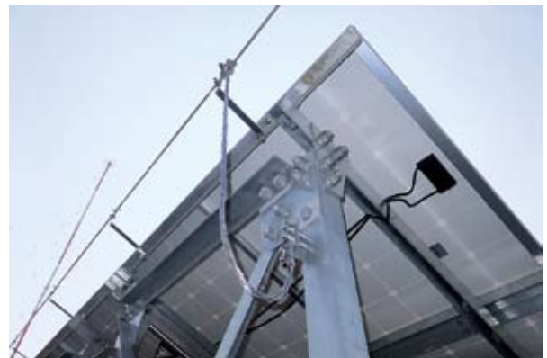
■ Photo 5: Lightning protection system for solar panels
