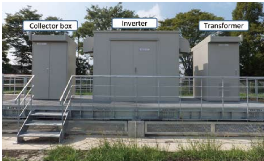
■ Photo 6: Cubicles for power supply equipment
