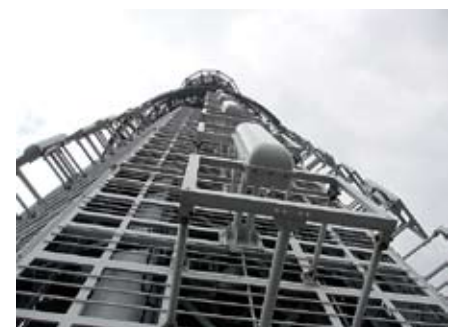
Photo 3: FM transmission antenna
