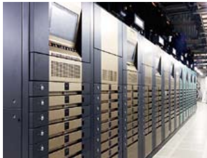
Photo 1: Television transmission equipment
